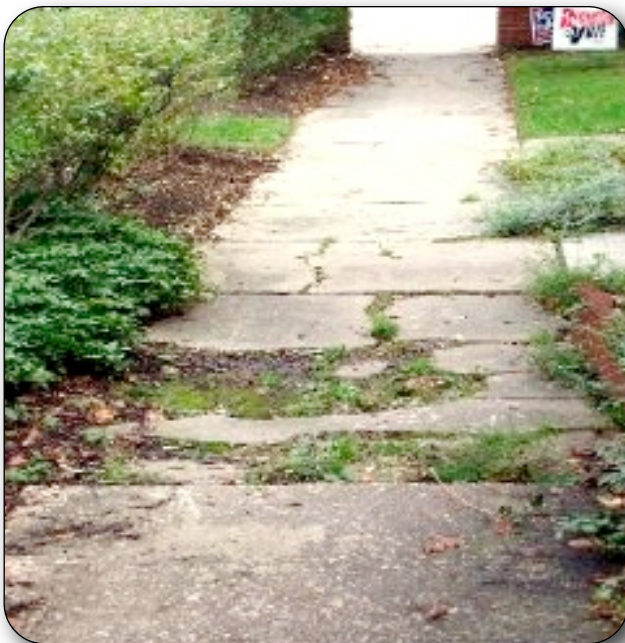
Cracking Sidewalk in Court #2
