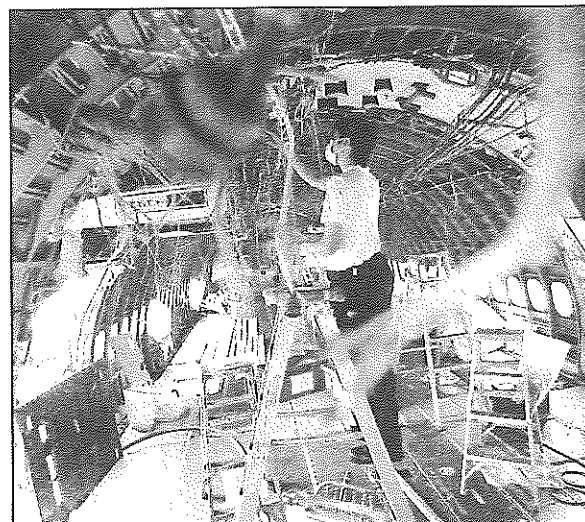
An aerospace technician rewiring the interior of a passenger plane to convert it into a freighter aircraft. The aviation and aerospace sector employs more than 18,000 people and has been growing steadily, driven by Asian demand. ST FILE PHOTO
